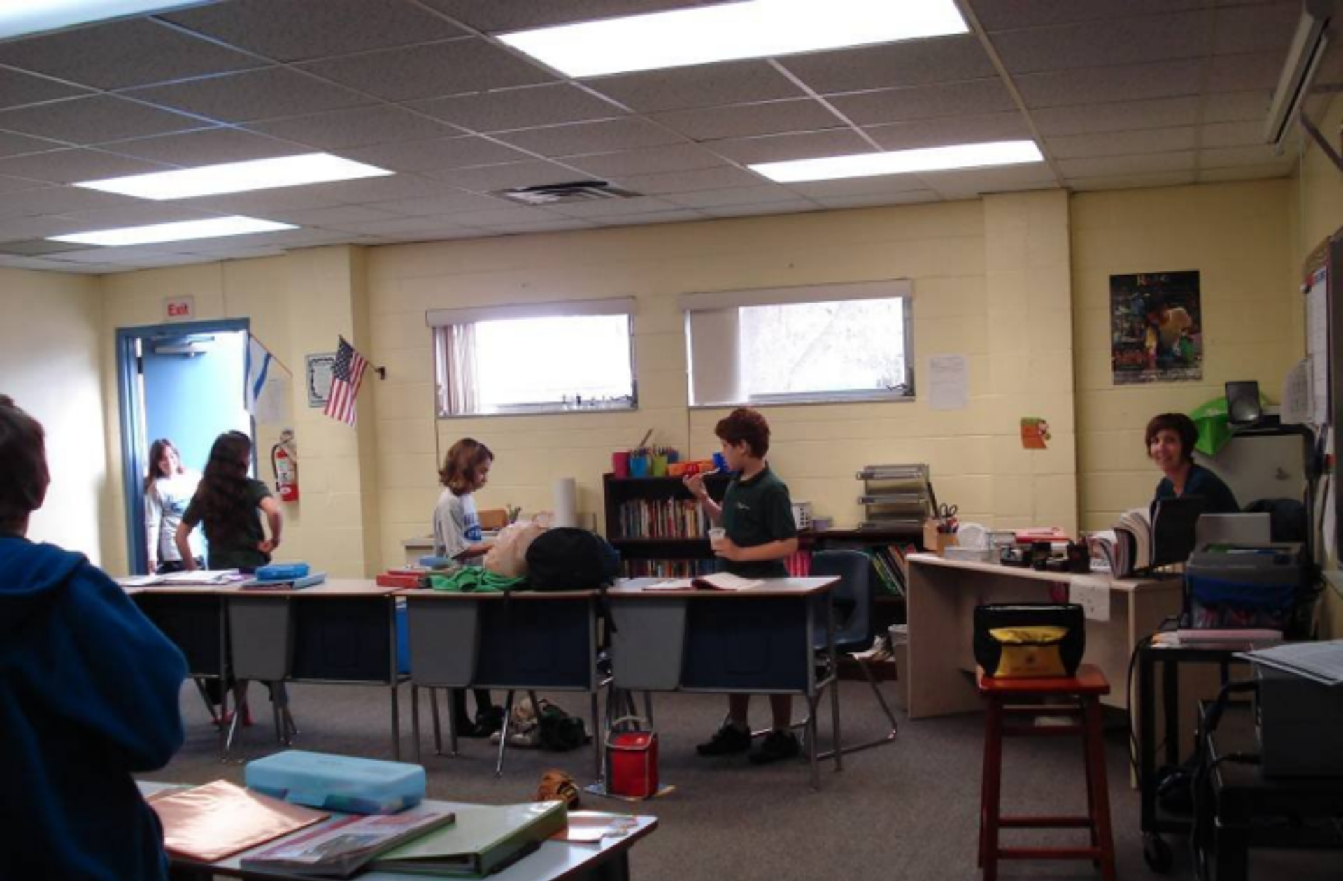
Before: Another typical classroom before the renovation - notice tiny windows - no daylight, no views, no fresh air, poor outdoor connections, non-ergonomic furniture, teacher work area contained within classroom. This is the area that has been converted into a student café (see next slide).
