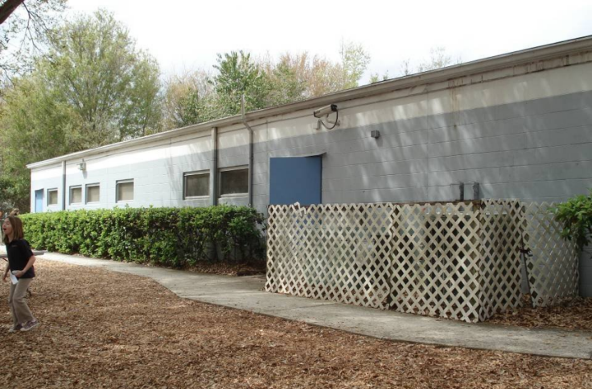
Before: This is the side of the intermediate school that faces a beautiful green playground and yet notice how the building takes no advantage of its setting. Small slit windows bring in little daylight and offer no views and there is no attempt to use the outdoors as an extension of the
